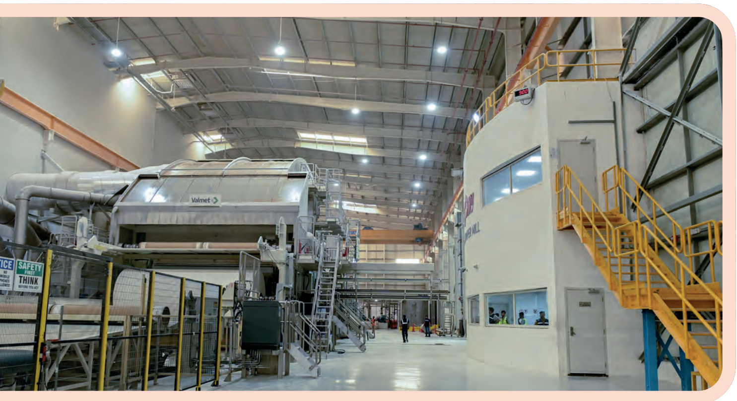
PM3 was commissioned in 2019: the company’s Valmet-supplied Advantage DCT 200HS line has a production capacity of 65,000tpy.
